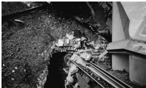
Another view of underbridge 79 from above with the derailed wagons hanging into the abyss created by the derailment.
