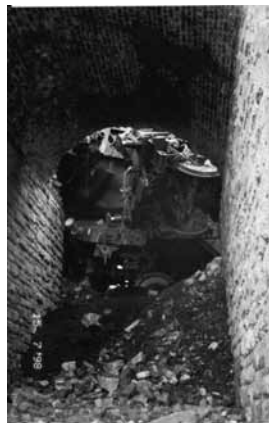
The view on the day after the derailment, Wednesday 15th. July, under underbridge 79 from the Down side showing how derailed coal wagons had smashed through the Up side of the bridge arch.
