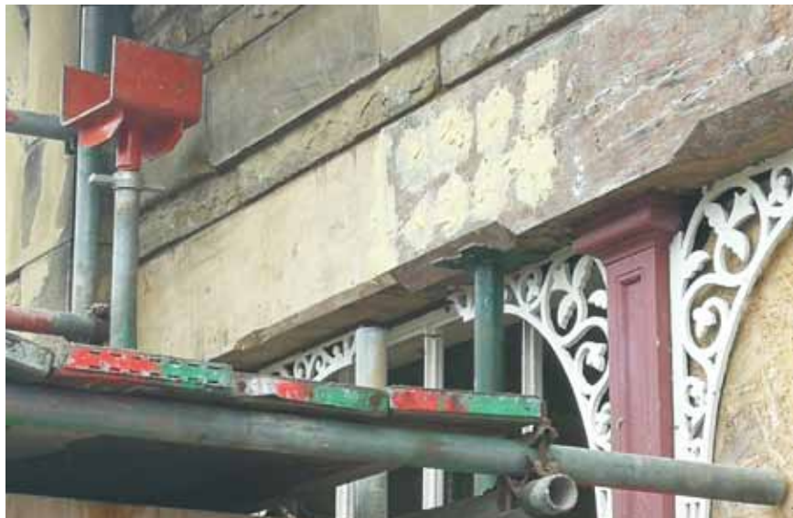
Acrow props support the defective lintel beam at Settle station.
