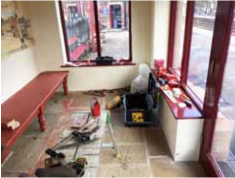
Above, above right and below: Ged Pinder and the Unit 8a team have been busy at Appleby constructing a Midland-style bench for the new waiting shelter.
