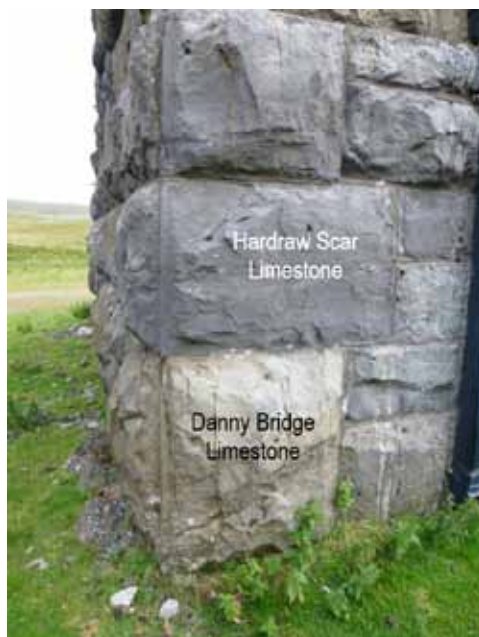
One of the few examples of Danny Bridge Limestone used in Ribbleshead Viaduct. Note the contrast in its colour with the darker, Hardraw Scar Limestone. Photo: Bill Fraser
